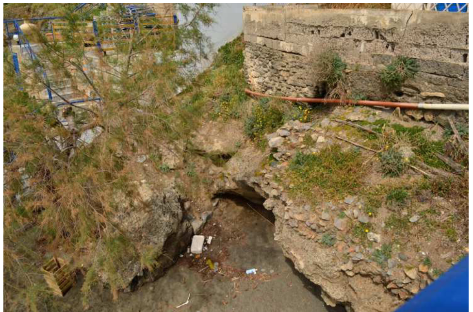
Fig. 38 Remains of coastal structures embedded into modern ones.
