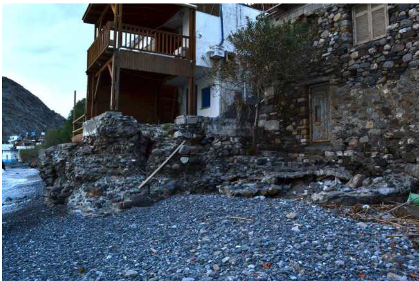
Fig. 36 Part of a coastal structure of uncertain function (E part of the beach).
