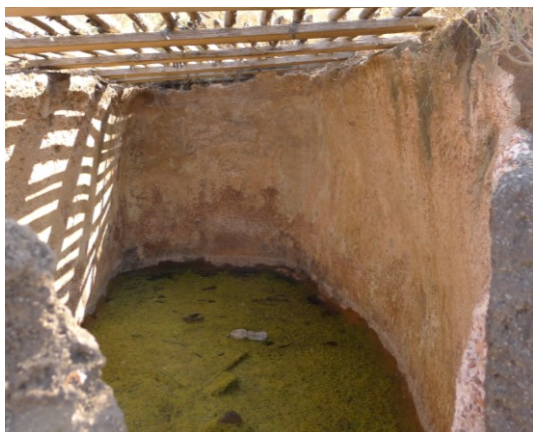
Fig. 21: la cisterna in UT1100.
