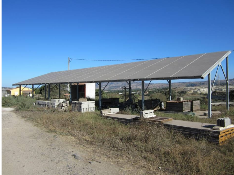
Fig. 8.4 – Rooftop photovoltaic system
