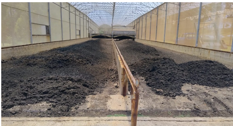
Fig. 60. Fresh sewage sludge deposited at the entrance of the two parallel channels.
