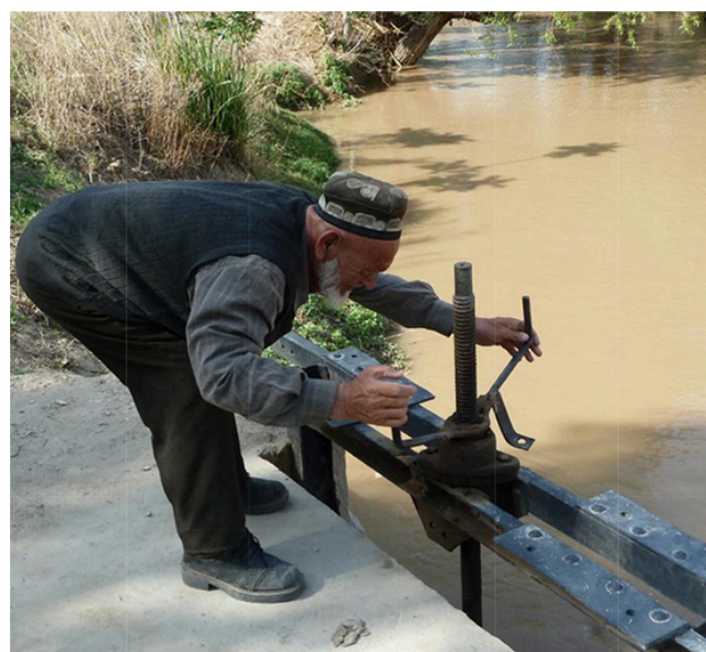
Fig. 7. Rehabilitation of water gates to improve distribution of irrigation water. The breakdown of obsolete water infrastructure caused immense water losses along the canals and the distribution systems in Tajikistan, Aral Sea basin (WOCAT entry n. 1444; https://qcat.wocat.net/en/wocat/technologies/view/technologies_1444/ ).
