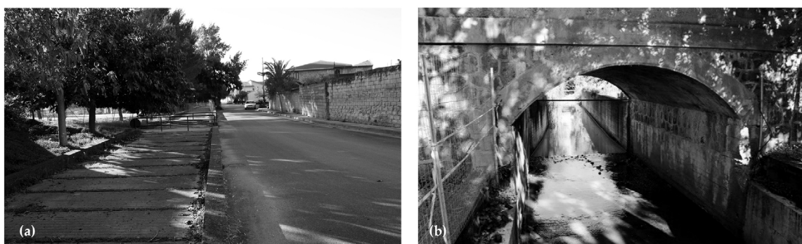
Figure 6. Tract of the culvert channel in the city center of Solarussa (a). Section of the channel in the intersection of two water infrastructures, natural and artificial one (b).
