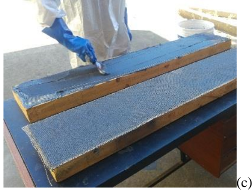
Fig. 3. Application steps of the reinforcement on a CLT specimen (a) flax fiber, (b) fiber positioning, (c) resin application.
